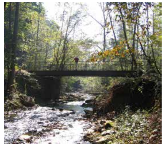
Former Executive Director and Current Council Member, Bill Clifton, stands at Fish Dam Creek Bridge
